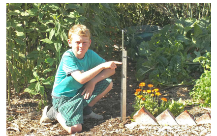
Each zone has a clear pressure monitor tube indicating the water pressure in the zone. Beau is pointing to the water level in zone 11 and the pressure is about 40 cm head of water.
