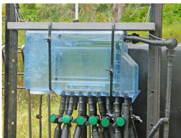
Water in flow-splitter has stabilized so the inflow matches outflow
