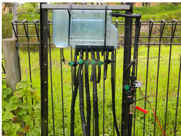
The inlet valve and the solenoid valve on the right
