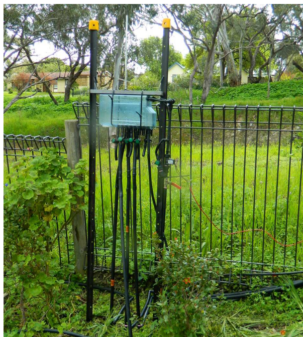
Flow-splitter mounted on star pickets
