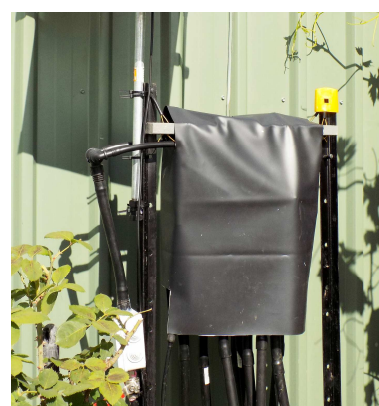
Light-proof cover protecting the flow-splitter
