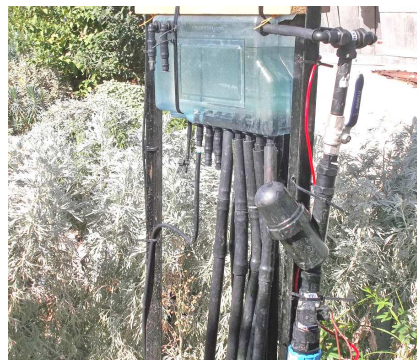
Flow-splitter delivering water to each of the eleven irrigation zones
